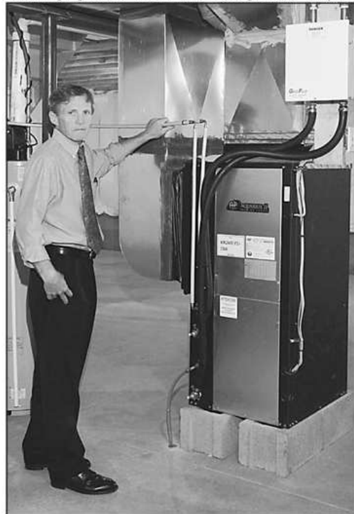
Larry Gurslin stands next to an Aquarius water convection system unit that can handle heating or cooling from a ground source heat pump. This unit is on the model home and is a green energy option on homes in Jim Beehler’s new senior housing development, Hamlin Meadows in Hamlin.
