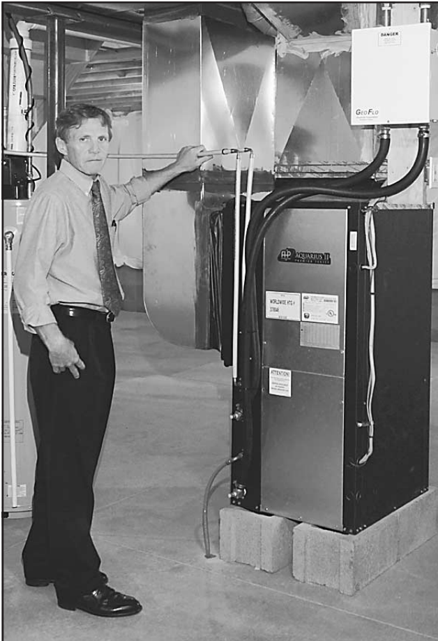
Larry Gursslin stands next to an Aquarius water convection system unit that can handle heating or cooling from a ground source heat pump. This unit is on the model home and is a green energy option on homes in Jim Beehler’s new senior housing development, Hamlin Meadows in Hamlin.
